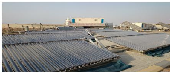
Figure 9: Solar absorption cooling installed at RAKRIC
